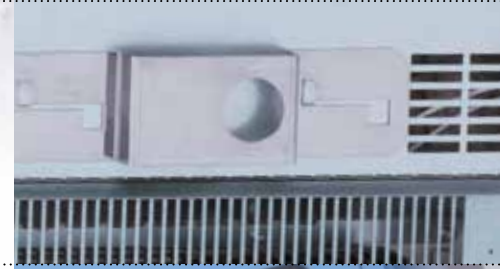
Fresh air damper provides control over air exchanges
