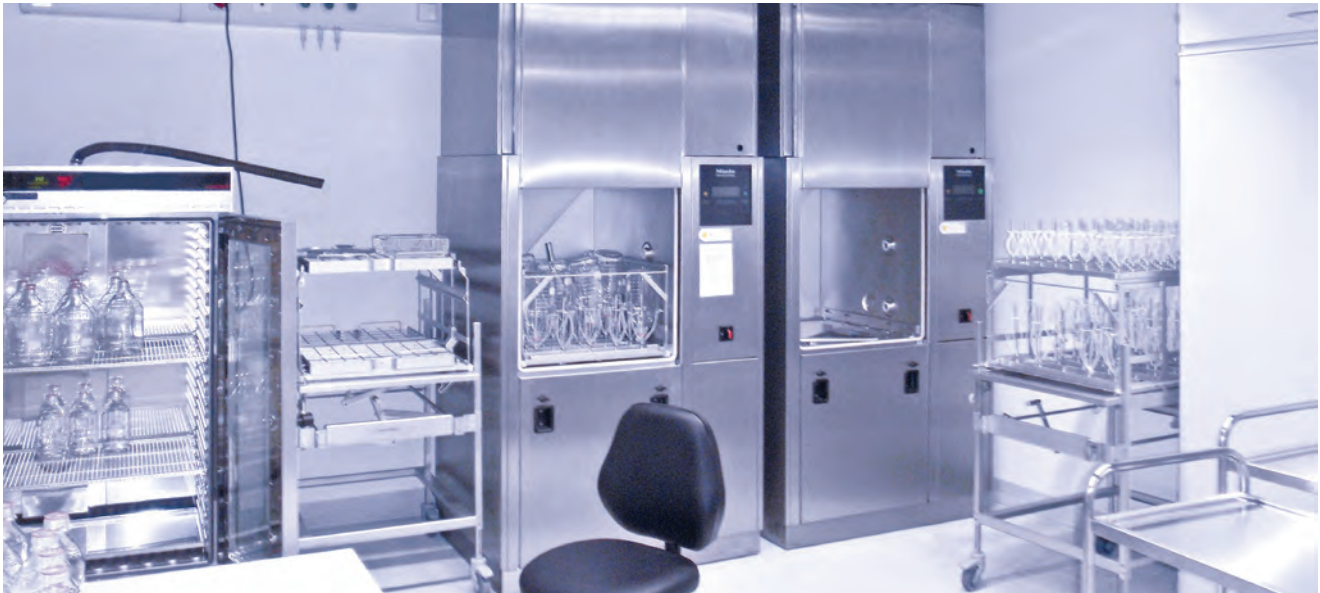
Central laboratory reprocessing room
